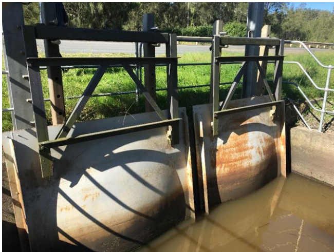
Figure 3-3 Pennington Drain flood gates
